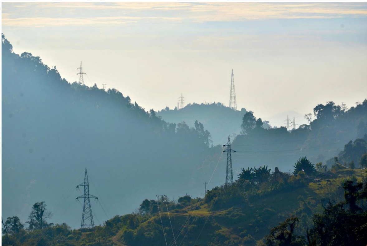
Image 4: Installation of power transmission lines entails clearing large corridor of forests. Photo: Thinley Namgyel.
