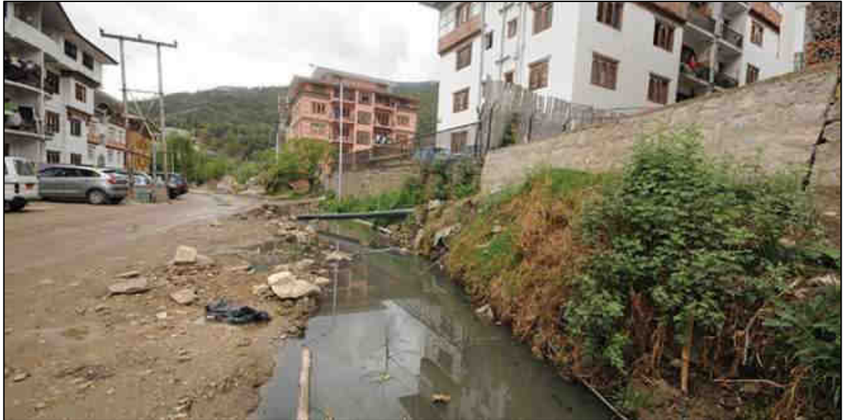
Figure 2-9 Septic tank leaks in Motithang (Source: Kuensel, 1 May 2018)
