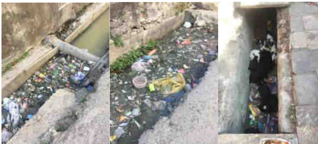
Figure 2-10 Solid waste dumped in drains around Clock tower, Thimphu
